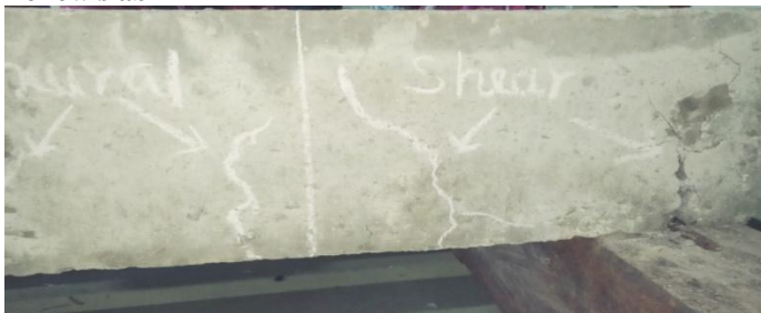
FIG 5.7 CRACKS ON HOLLOW-CORE SLAB
